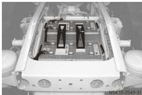
Example: batteries between the longitudinal frame members
